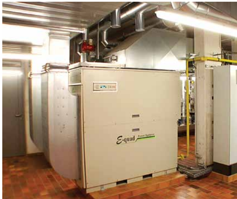
Two natural gas Capstone C65 microturbines make up the combined heat and power system at Catholic Hospital Koblenz in Augsburg, Germany.
