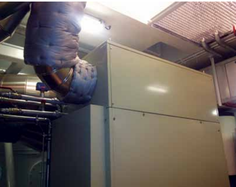
Two liquid natural-gas fueled Capstone C30 MicroTurbines onboard the MTS Argonon Type C tanker in Rotterdam, Netherlands, operate in an N+1 setting and serve as the main electrical power supply.
