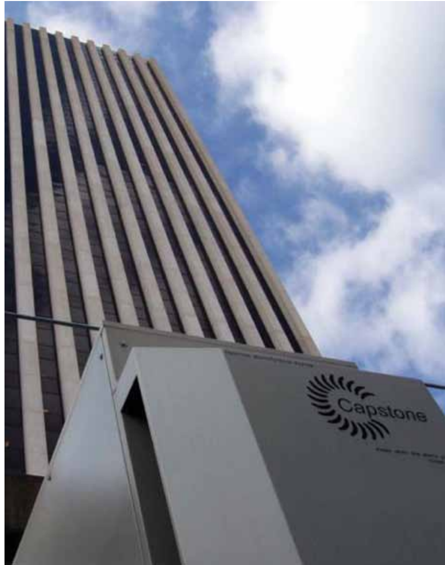
Six Capstone C60 microturbines assure power security at this downtown Houston site.
