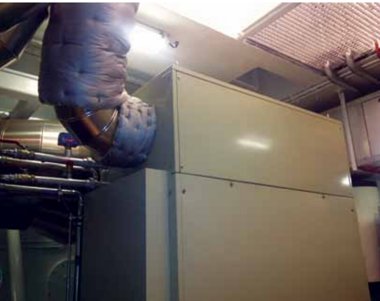
Two liquid natural-gas fueled Capstone C30 MicroTurbines onboard the MTS Argonon Type C tanker in Rotterdam, Netherlands, operate in an N+1 setting and serve as the main electrical power supply.
